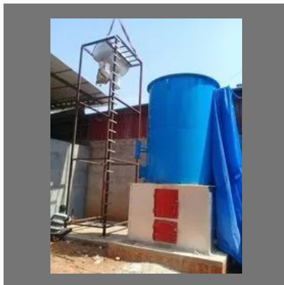
Wood Fired Thermic Fluid Heater
