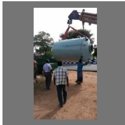
Industrial Water Softener Plant
