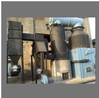
Wood Fired Thermic Fluid Heater
