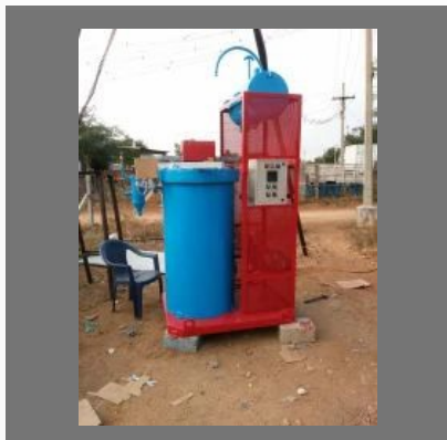
Hot Water Boilers
