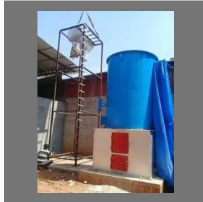
Thermic Fluid Boiler
