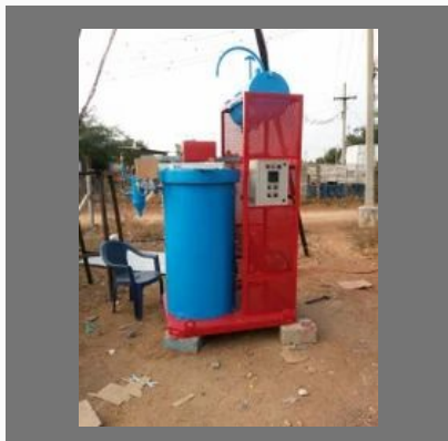
Package Steam Boiler
