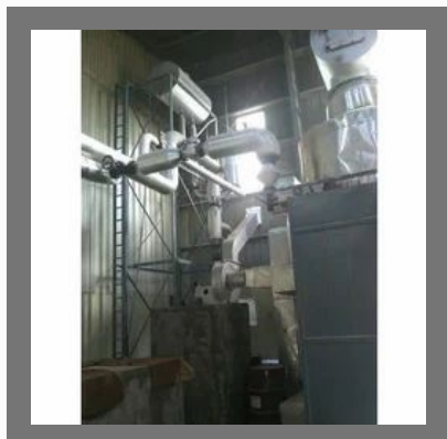
Thermo Pak Boiler
