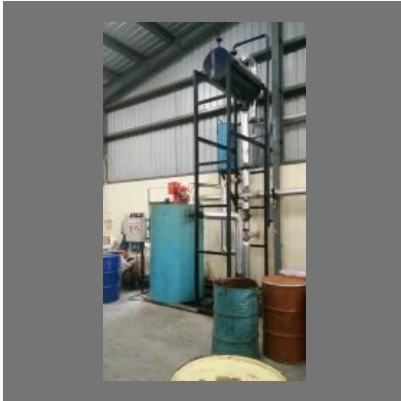
Thermic Fluid Heater Diesel Gas Fired
