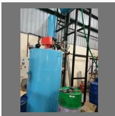
Thermic Fluid Heater
