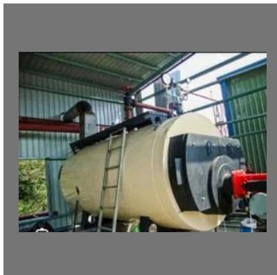
Diesel Fired Steam Boiler
